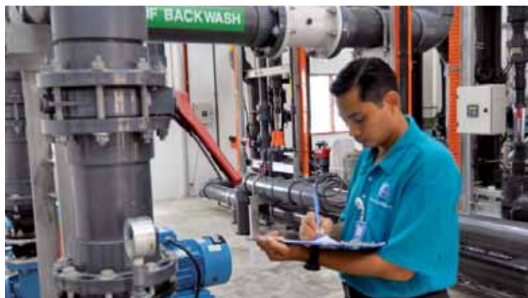
◀ Scheduled maintenance is strictly adhered to at all our WTPs
