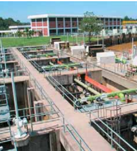
Raw water intake at SSP2 WTP
