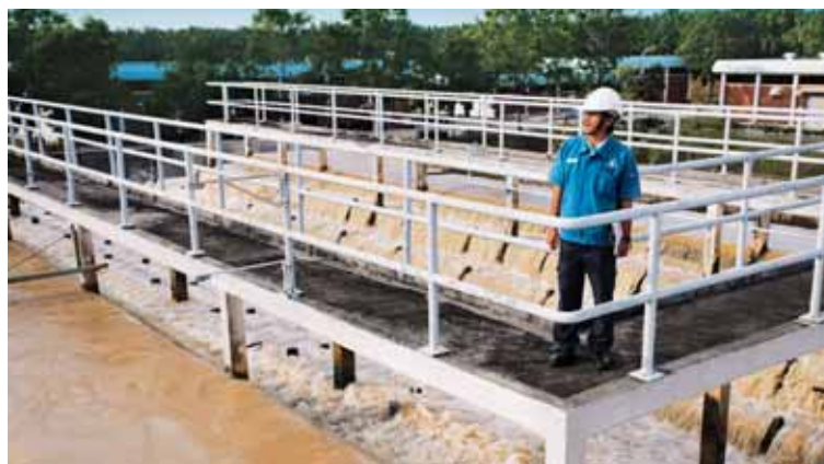
◀ Aeration process to oxidize the raw water at SSP2 WTP
